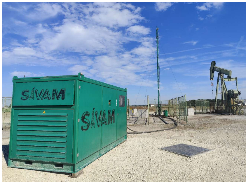
Fig. 1 – General installation layout of the PowerLift PL600-C100 hydraulic unit on the well
